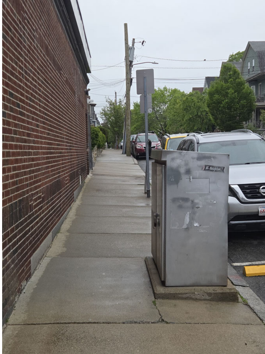
Figure 4. Ball Square cabinet, viewed along the sidewalk.
