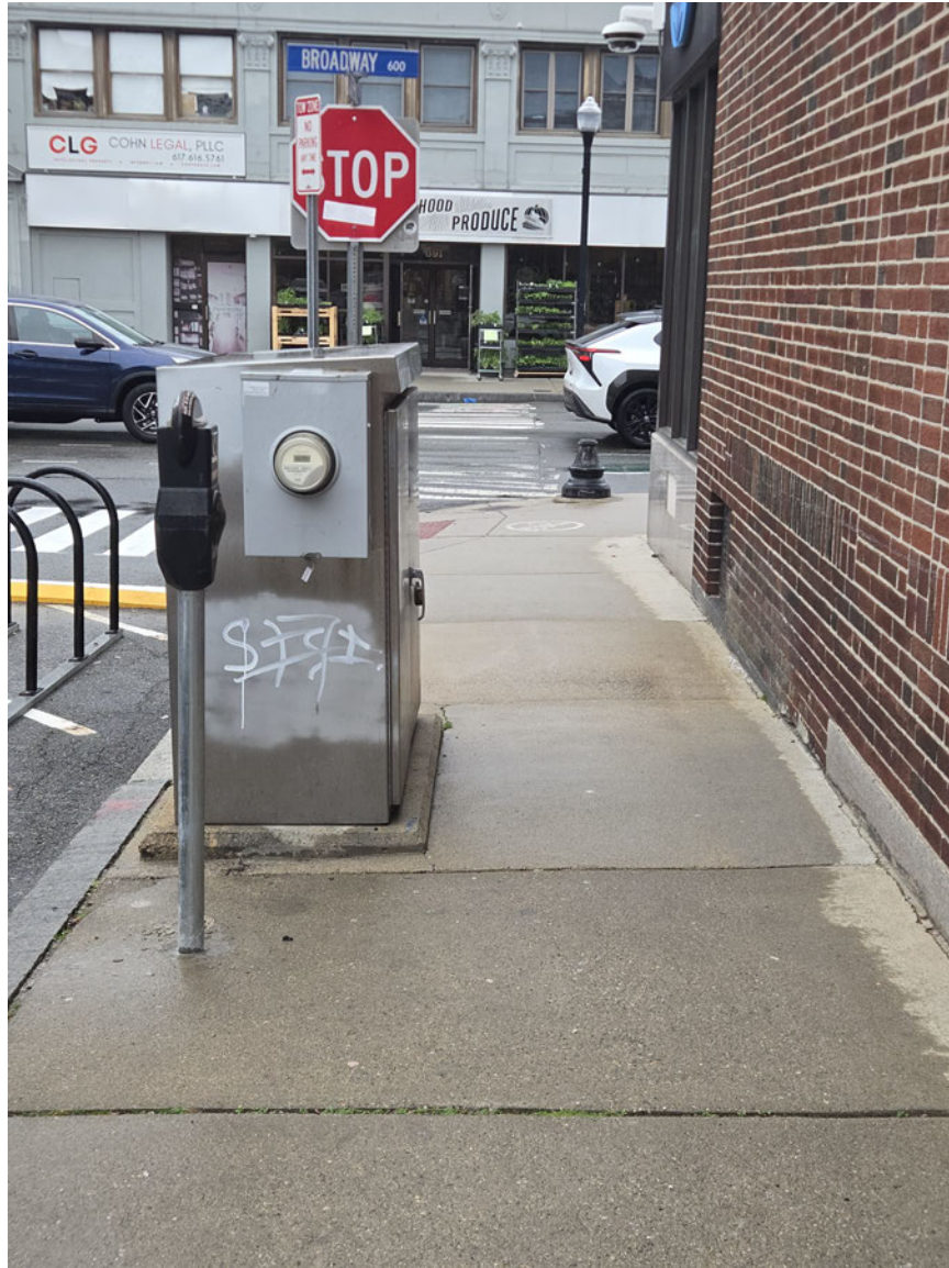
Reverse angle of the same cabinet, looking toward the Broadway/Josephine corner. The weathering and graffiti are visible evidence that this cabinet predates the MassCEC EV charging program. The wider commercial sidewalk and the parallel parking configuration are also visible — conditions that do not obtain at 135 Hudson Street.
