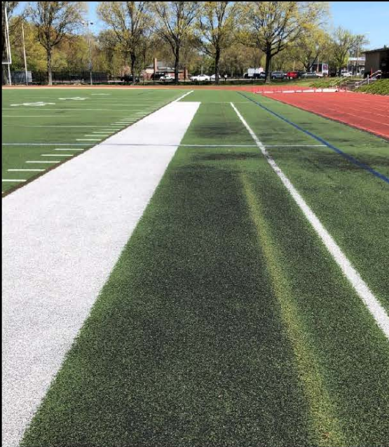
Synthetic Turf Surface in poor condition
