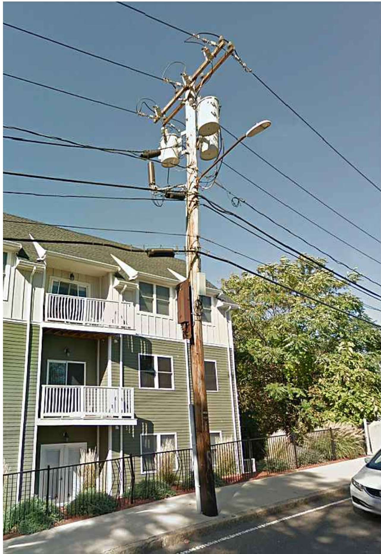
UTILITY POLE – BEFORE
