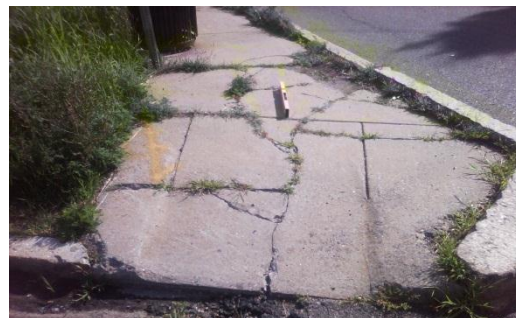
Poor ramp in need of Full Replacement
