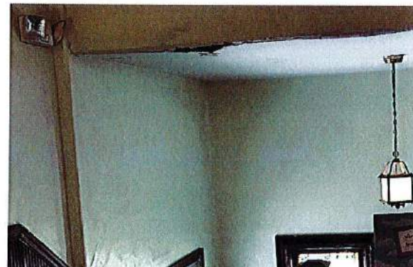
3 Roof-wall intersection and possible leak above the north stair.
