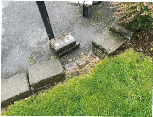
Older unit block walls in need of replacement
