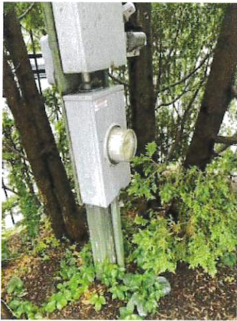
Utility area overgrown.
