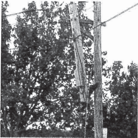
Natick and Framingham have filed home rule petitions that would allow the towns to fine utility companies for leaving double poles like this in place after a certain period of time.
