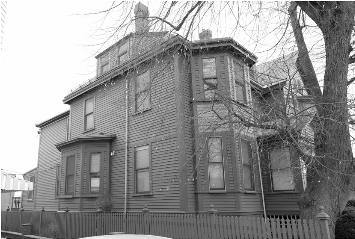
Photo 6. View of left (northwest) side elevations, and front (southwest) elevation (partial), looking northeast.
