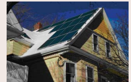
Residential Solar Panels installed by Sunbug Solar in Somerville.
