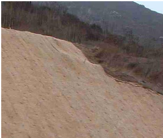
Straw is for horse bedding, not erosion control or slope landscaping. A straw blanket/mat slope before the rain.
