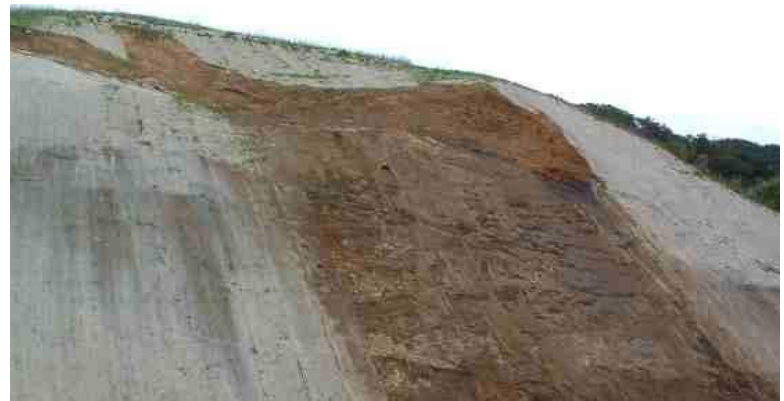
Straw mat hillside sliding away after a few light rainfalls. Should have been terraced with cross drains, mulched and planted.
