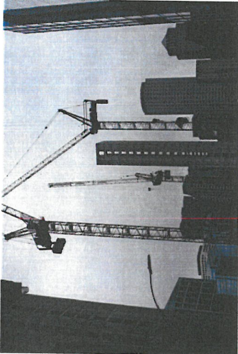
Construction underway on One Seaport Square which is opposite the Stables Federal Courthouse. It will be housing and retail.
