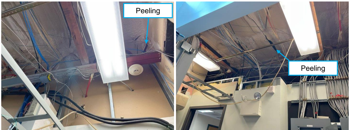
Photo 6 - Spray-foam insulation installed at underside of roof deck, as shown in the Electrical/IT room, is peeling and not continuous.
