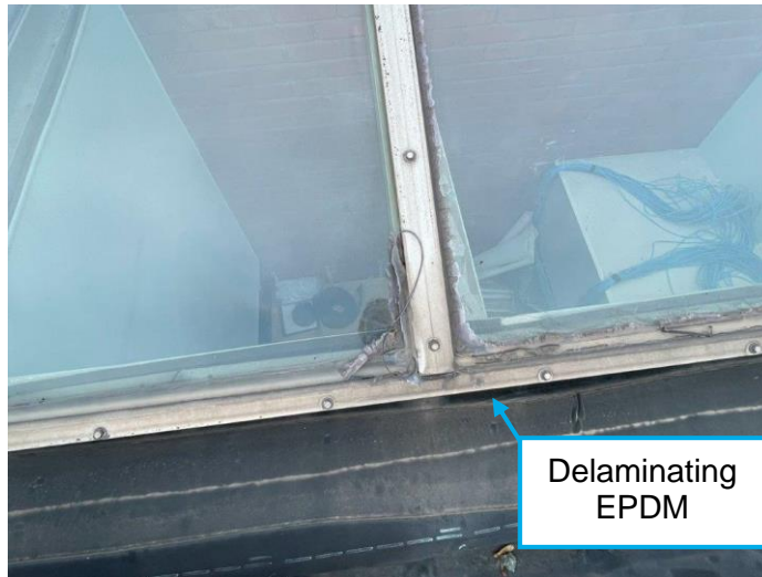
Photo 5 – Sloped skylight at West elevation. EPDM membrane is delaminating at skylight curb.
