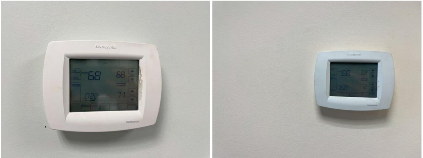
Photo 20 - Honeywell thermostats and settings at reception (left) and open office area (right).
