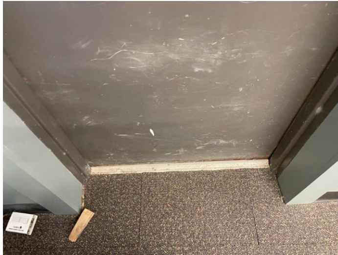
Photo 9 - Back egress door. Occupant seated near egress door has noted draftiness. Evidence of moisture damage is apparent at door head. Blower door test showed 123 CFM air leakage at egress door when tested at @-50Pa. Refer to Appendix D.
