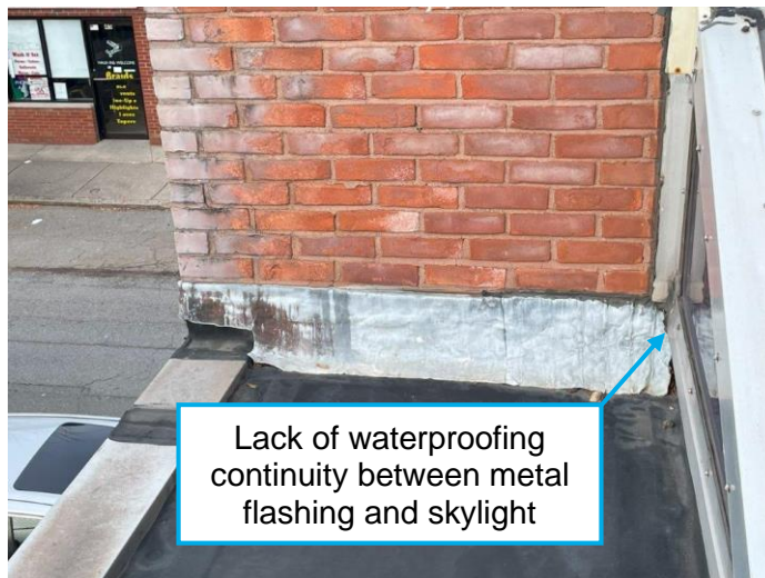
Photo 4 - Metal flashing at parapet. Low flashing height. Rough edges of flashing are touching the roof, which may cause punctures in the EPDM membrane. Flashing is not tied into skylight, relying only on sealant, and creating potential for water penetration at corner joint.
