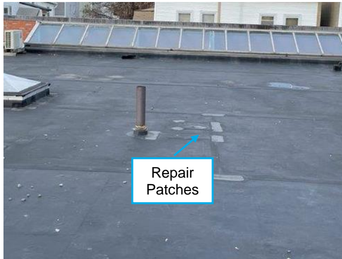
Photo 3 - Isolated areas of repair patches on EPDM roof.
