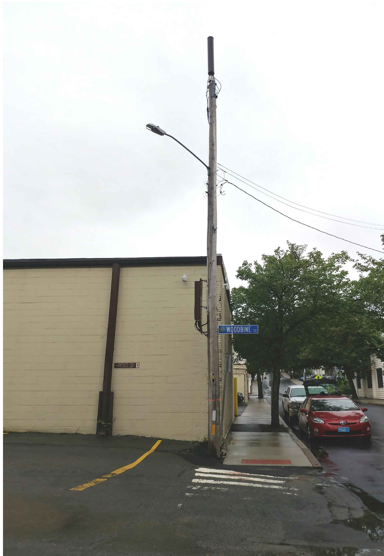
UTILITY POLE – BEFORE
