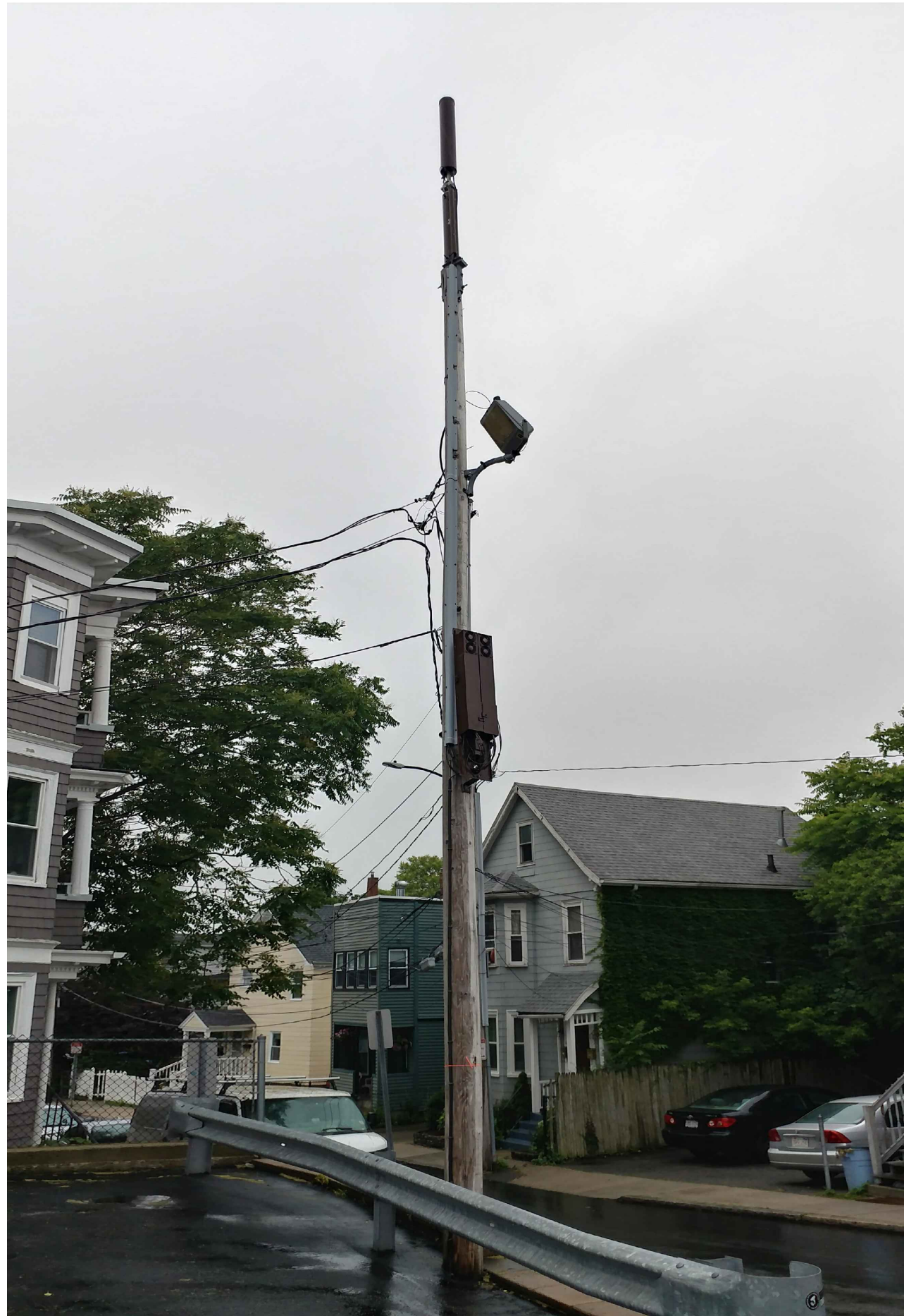
UTILITY POLE – BEFORE
